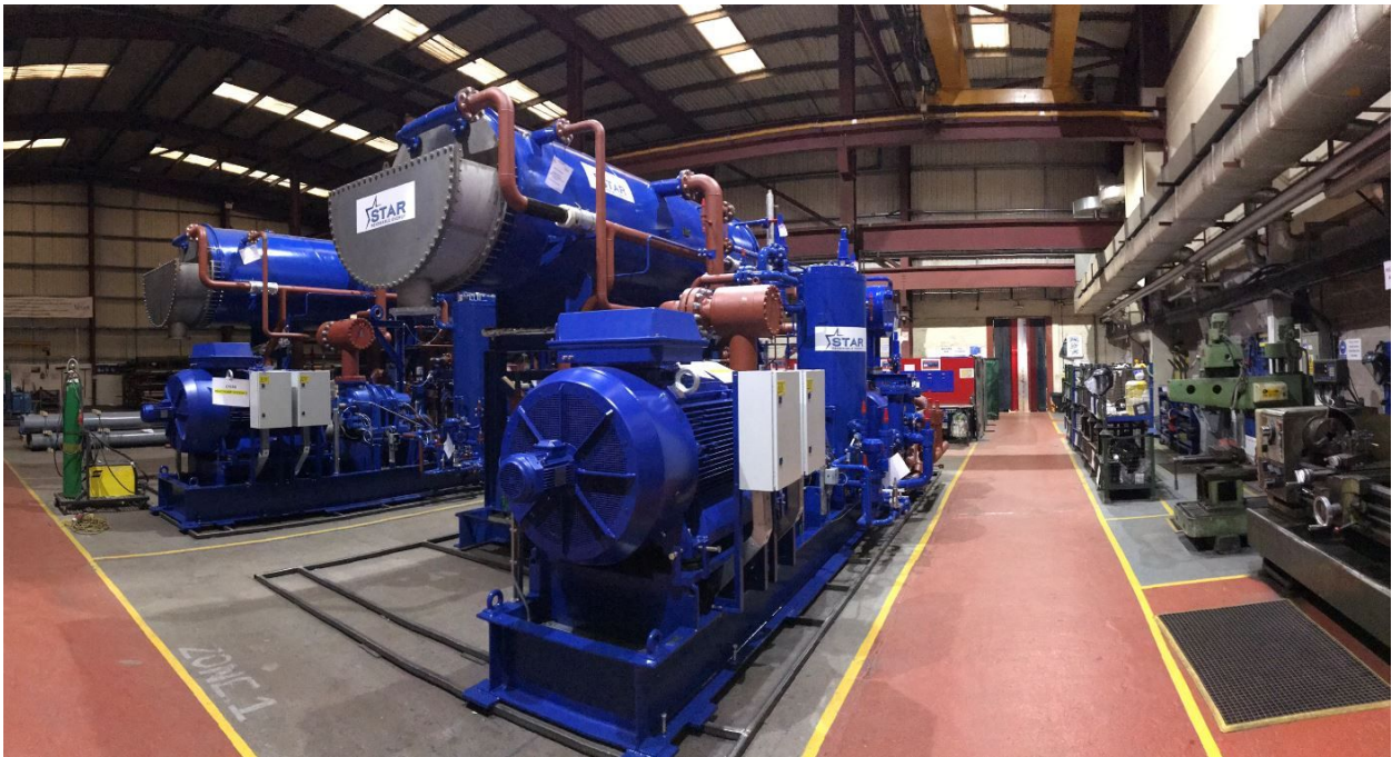
Figure 6 Star Renewable Energy - Queens Quay Heat Pumps
