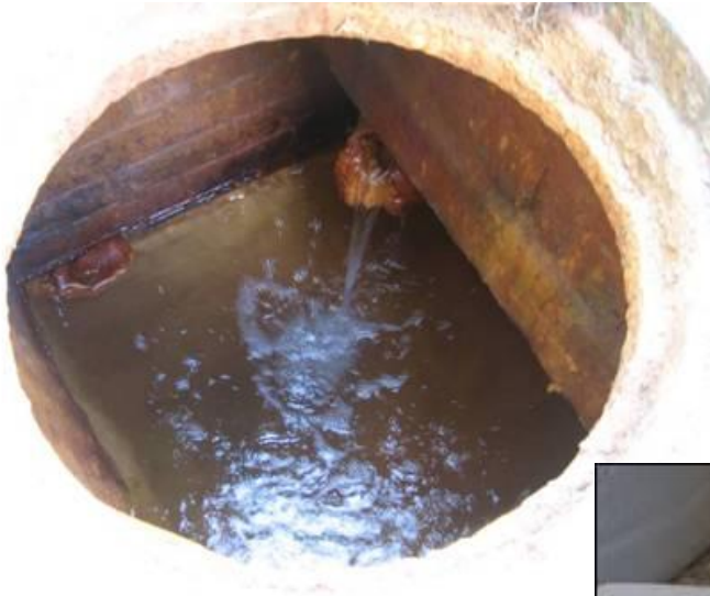
Lumphinnans (clogged reinjection well) See Banks et al (2009) Doi: 10.1144/1470-9236/08-081
