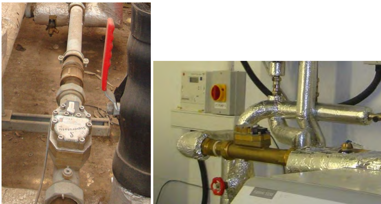
Figure 68 – Incorrectly mounted vortex flow meters
