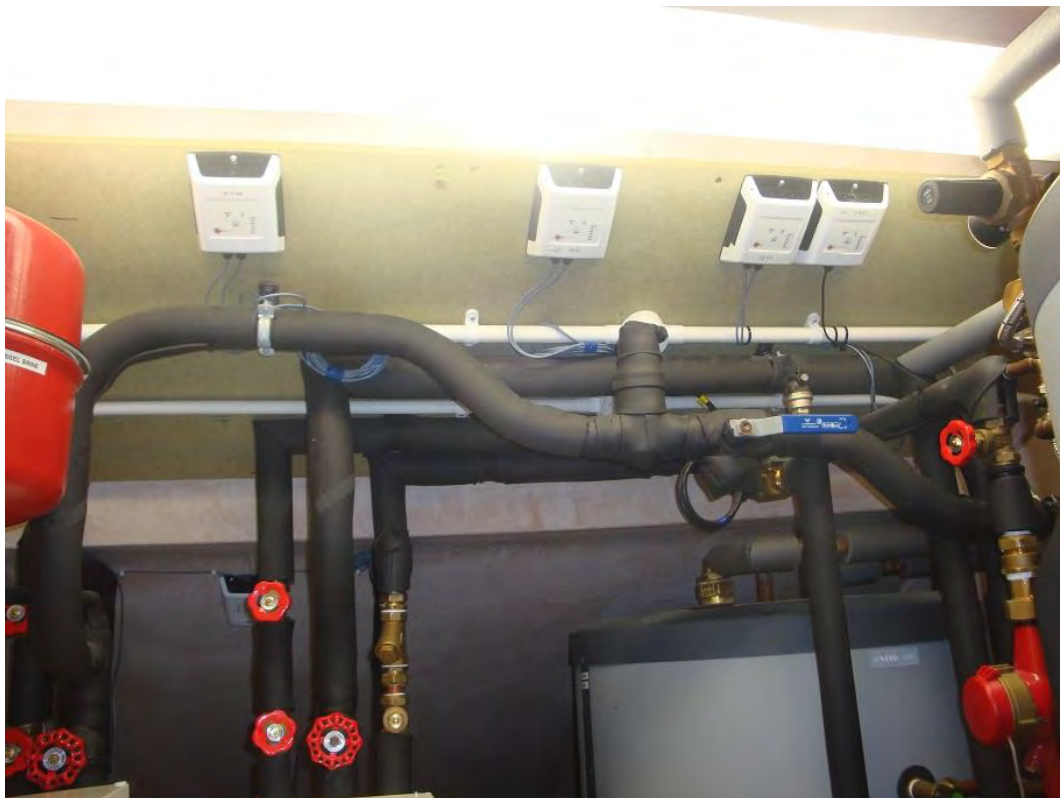
Figure B 11 – TES-32 temperature sensors mounted on the ceiling of a plant room.
