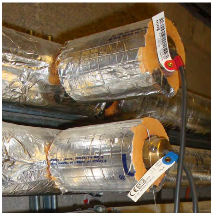
Figure 62 – Incorrectly designed sensor fittings
