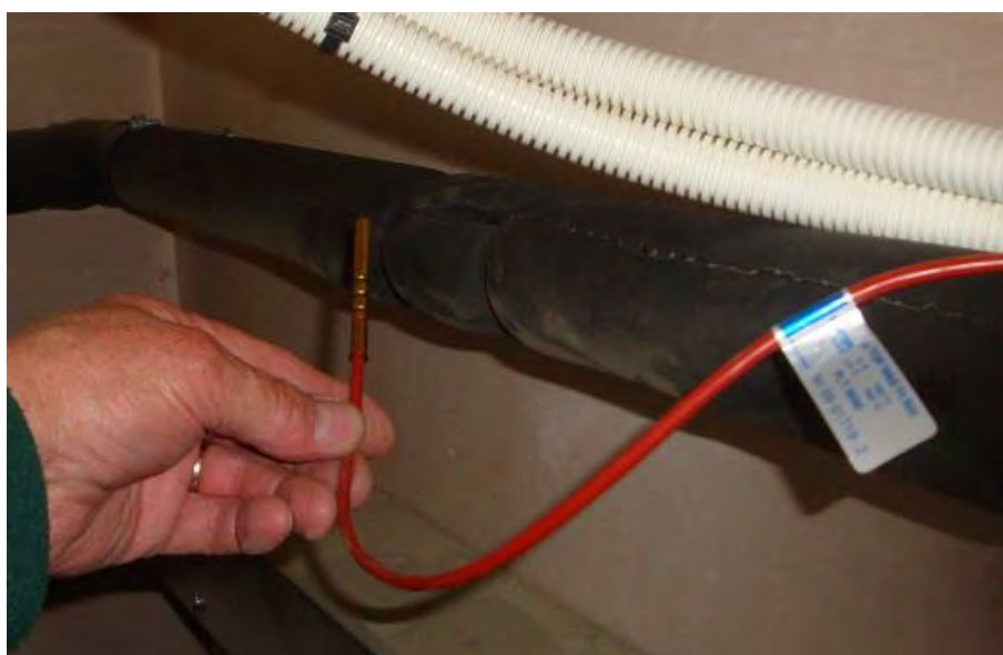
Figure 65 – Loose temperature sensors on the wrong pipes
