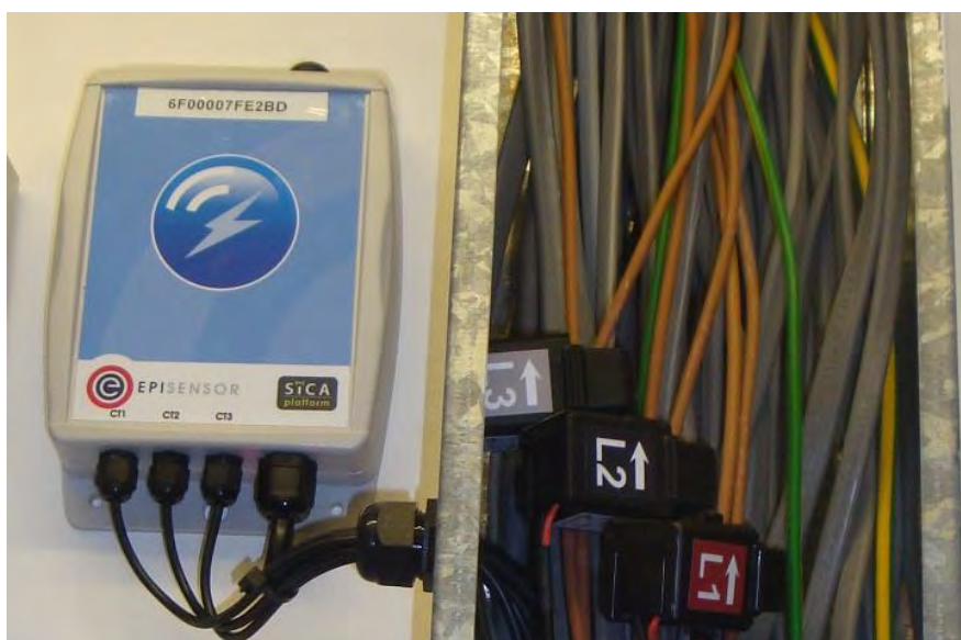
Figure B 7 – ZEM-61 3-phase electricity monitor with current transformers installed in cable trunking.
