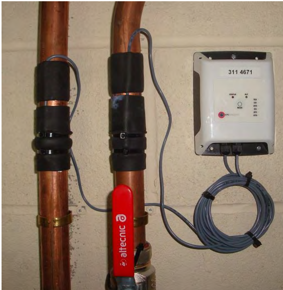
Figure B 12 – Temperature probes attached to copper pipes.
