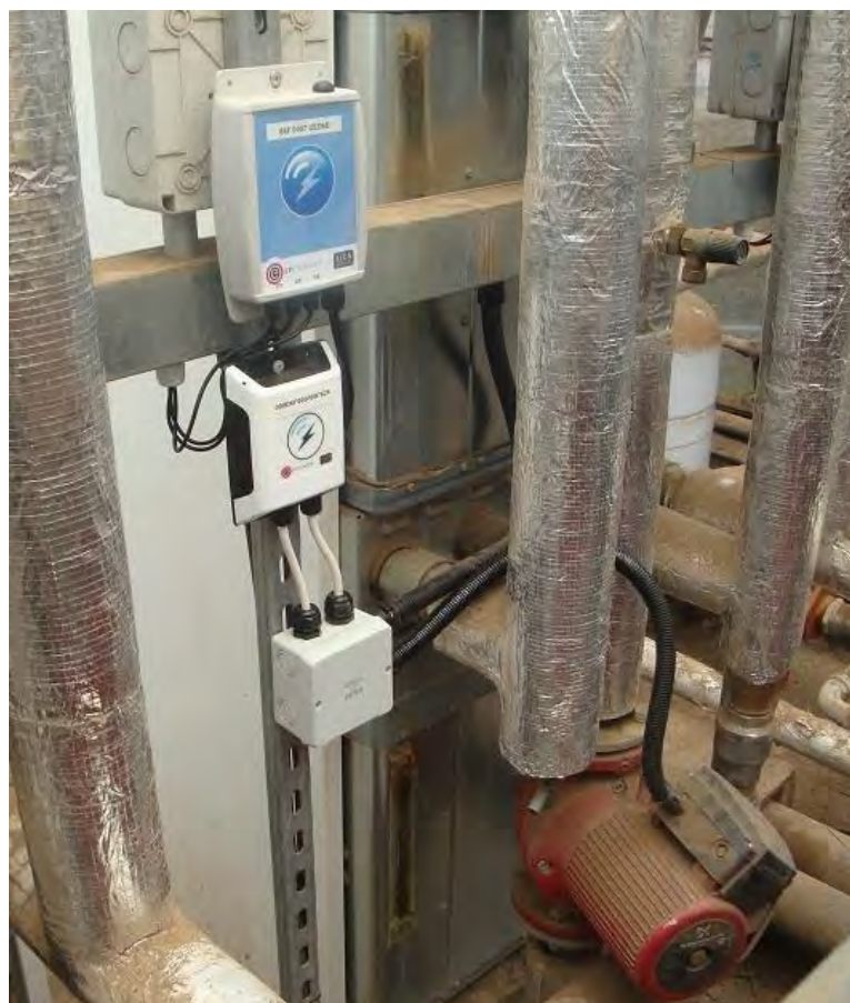
Figure B 9 – ZEM-61 and ZEM-30 monitors on a heat pump
