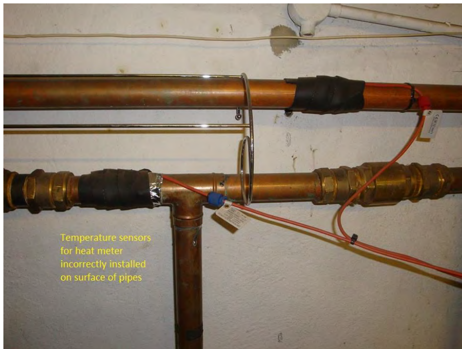
Figure 64 – Strapped on temperature sensors
