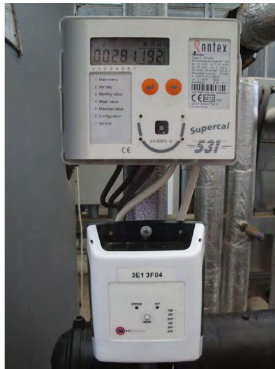
Figure B 15 – ZHM-20 M-Bus monitor connected to a Sontex heat meter
