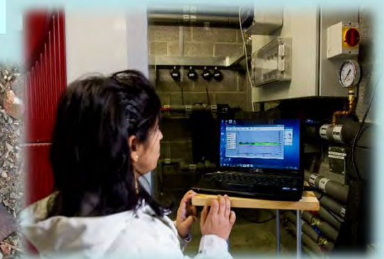
System data acquisition at site
