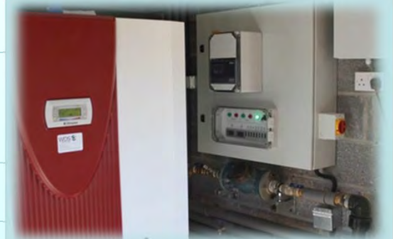
Heat pump with data collection and logger system
