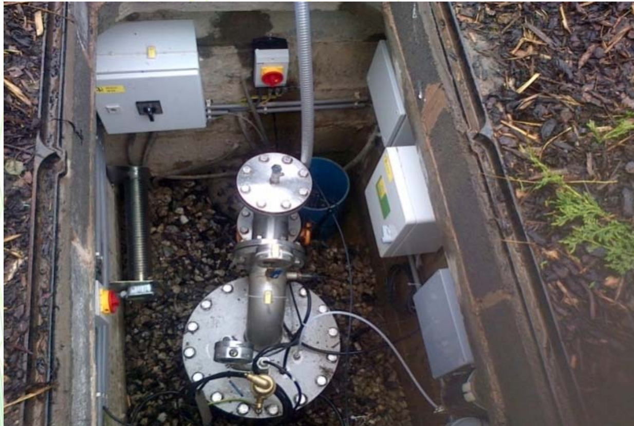
Below Ground Well Housing
