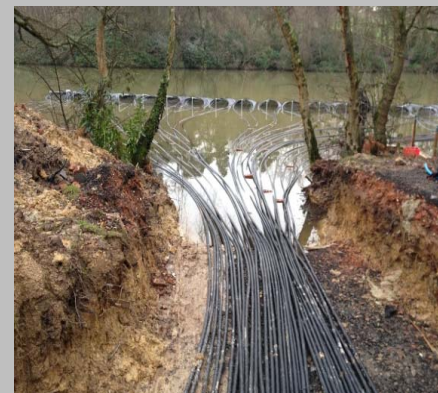
Collector pipe from 18 loops
