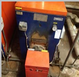
Old Oil Boilers
