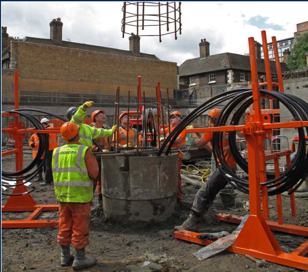
Loops fixed on outside 52m deep on full depth cage Placed under bentonite
