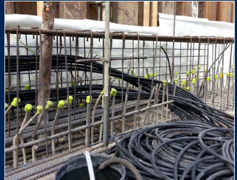
Loops at central collection point
